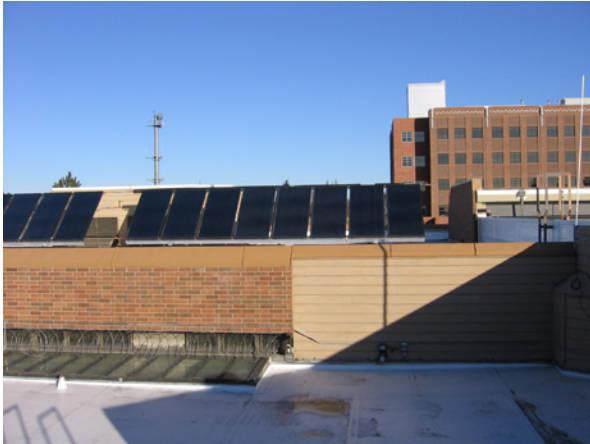
Solar roof at Clark County Jail
